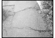
Cracked footway in Huddlestone Road
